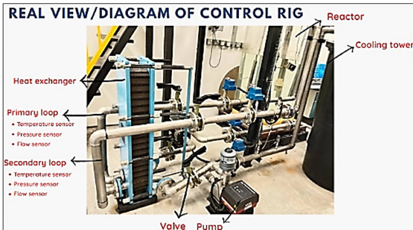
Figure 1. Real view of the process control rig for the RTP cooling system
